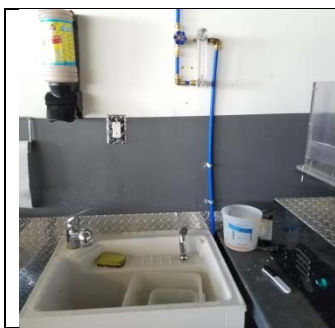
Example of a Flow Regulator and Shower Head Rinse Apparatus
